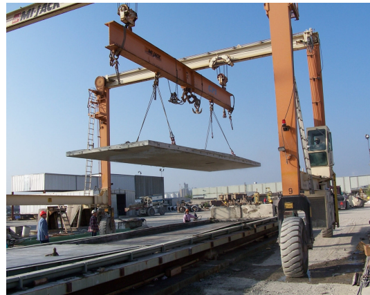
Moving a panel from the forms into storage for the Missouri project.
